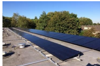
Brede School Zaltbommel 200 panelen
